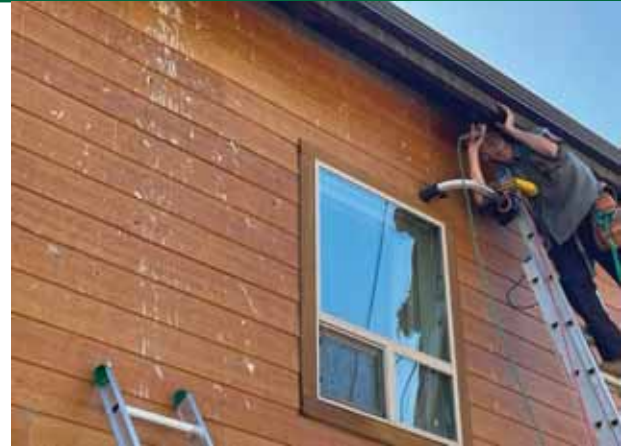
Above: 72-year-old Barry, installing hardware wire to keep the bats out of our Williams Grange attic and installing new bat boxes as an alternative housing resource for the bats.
