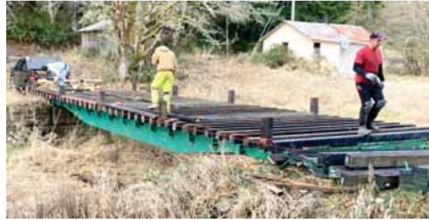
Below: Laying and attaching the 6x6 inch timbers on to the rail car base of the bridge.
