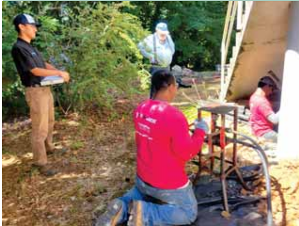
Above: Members of the Ram Jack crew working on Abernethy Grange hall.
