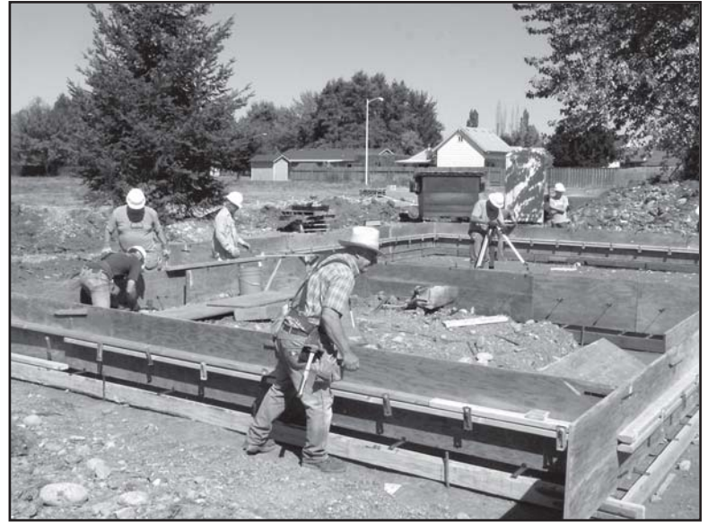
Clarkes Grangers and other volunteers set up concrete forms to prep for foundation installation
